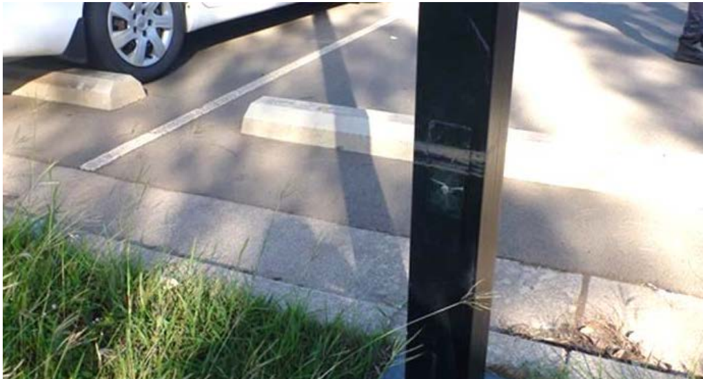
Figure 3.6 FLOOD DEBRIS LINE IN COUNCIL CAR PARK POST TC-MARCIA, BILOELA
